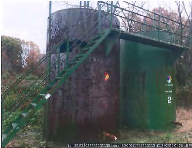
Photograph of heavily corroded brine tank. Large holes were present in brine tank 1. Brine tank 2 was less corroded, but small holes were observed.
