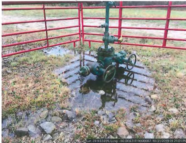
Photograph of the well head. The well head was leaking at the time of inspection. Gas was bubbling through rain water around the well head.
