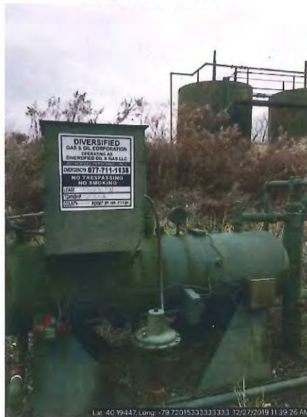
Photo #8 Information Placard and associated Production Equipment
