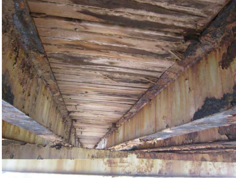
Photo 19 - Skinnners Falls Bridge: Typical deck underside condition. Note missing clips
