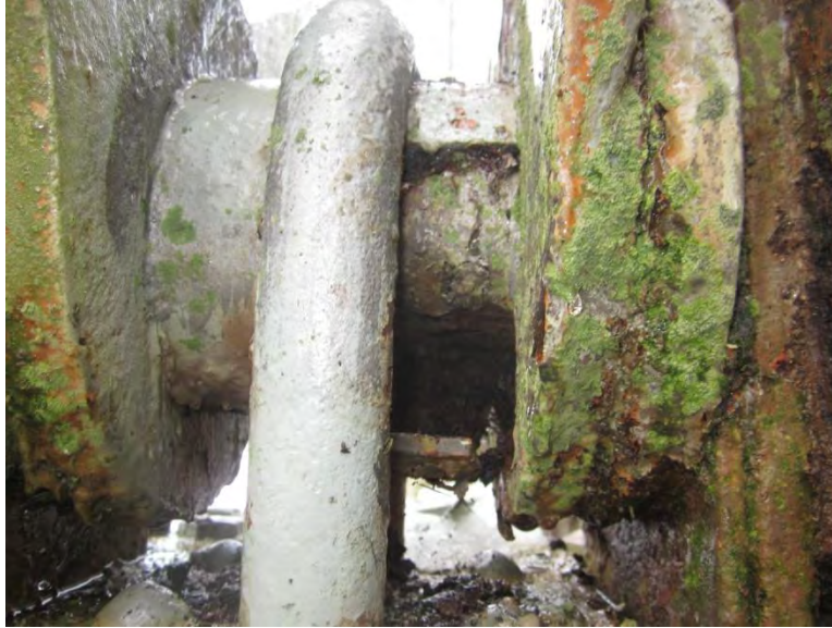
Photo 17 - Skanners Falls Bridge: Span 1, Left Truss, Panel Point L6 pin sleeve broken (Looking Ahead)
