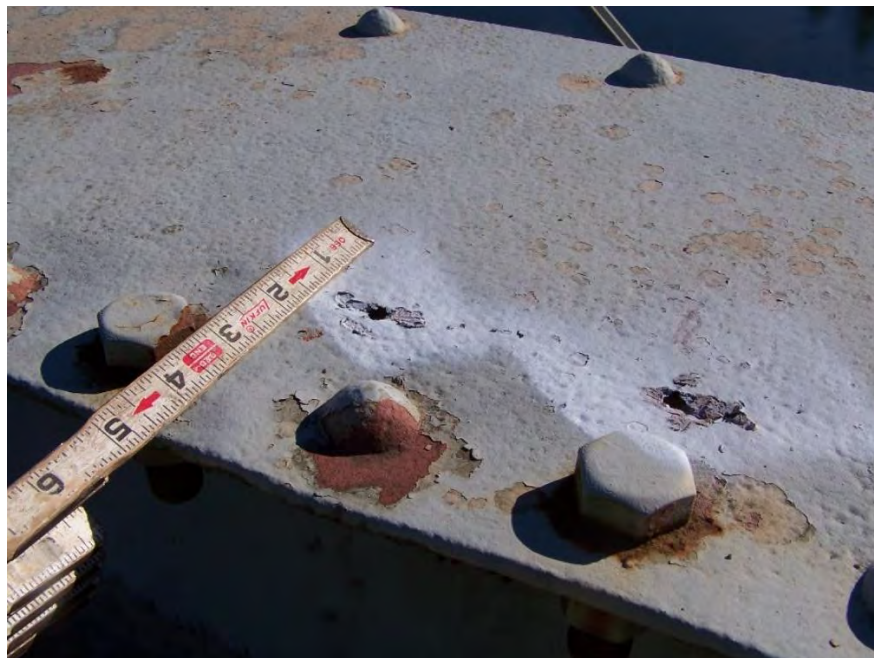
Photo 10 - Skinnners Falls Bridge: Left Truss Top Chord section loss
