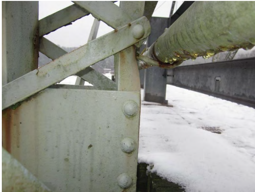
Photo 12 - Skinners Falls Bridge: Collision damage to vertical members at deck level behind the bridge railing
