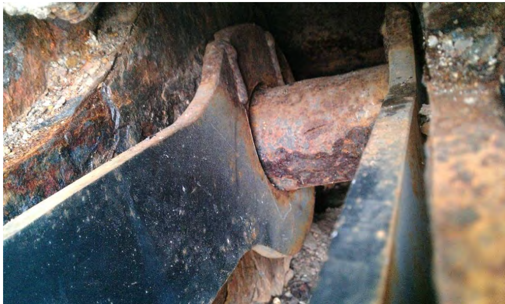
Photo 16 - Skinners Falls Bridge: Existing field welded s to lower chord forged eyebar heads
