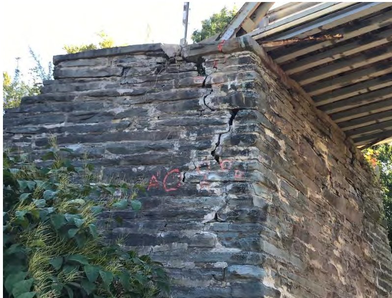
Photo 24 - Skinners Falls Bridge: Far Left Wingwall with Crack Monitoring Points and Full Height Step Cracking
