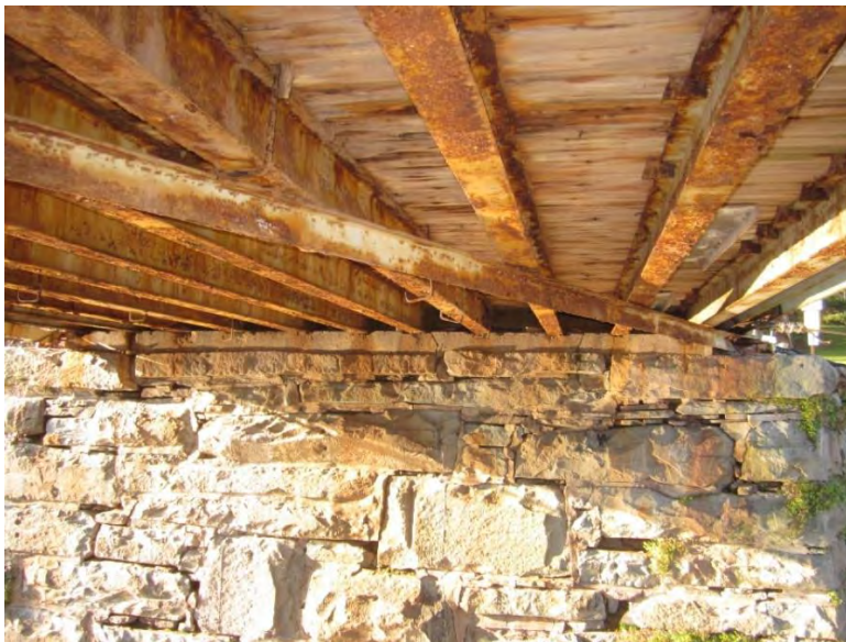
Photo 26 - Skinners Falls Bridge: Near Abutment with wide mortar joints with deep voids at the top half
