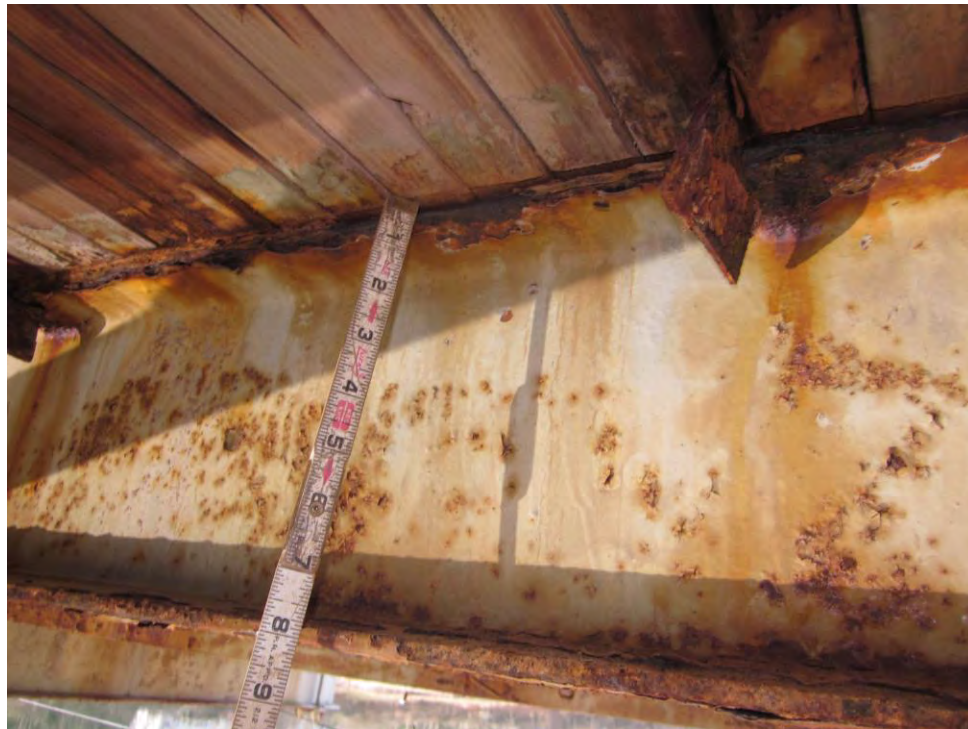
Photo 20 - Skinnners Falls Bridge: Gap between stringer and deck due to section loss
