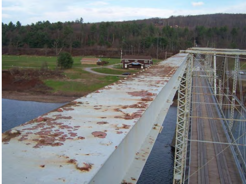
Photo 9 - Skinnners Falls Bridge: Left Truss Top Chord flaking paint and minor surface rust
