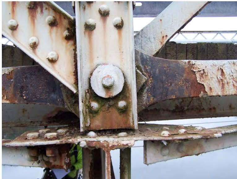
Photo 14- Skinners Falls Bridge: Span 1, Right Truss, Panel Point L8 retrofit pin cap (Looking Left)
