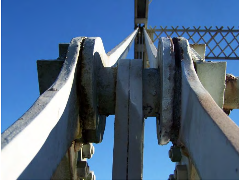
Photo 13 - Skinners Falls Bridge: Typical losses to eyebar heads at middle panel points
