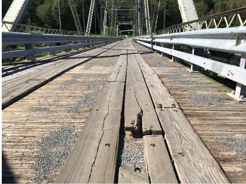
Photo 5 - Skinnners Falls Bridge: Timber Running Board Deterioration
