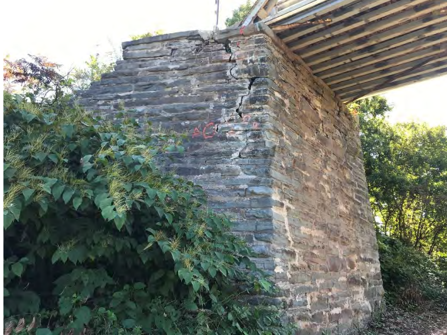
Photo 23 - Skinners Falls Bridge: Far Left Wingwall with Crack Monitoring Points and Full Height Step Cracking
