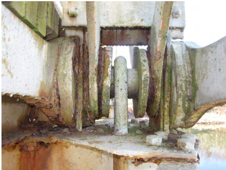
Photo 18- Skanners Falls Bridge: Span 2, Left Truss, Panel Point L6 extensive pack rust (Looking Back)
