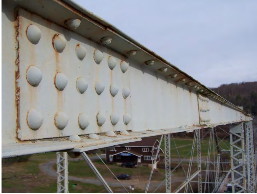
Photo 11 - Skinners Falls Bridge: Bent and misaligned bolts in top chord splices in Span 2 resulting in displacement of top chord channels.
