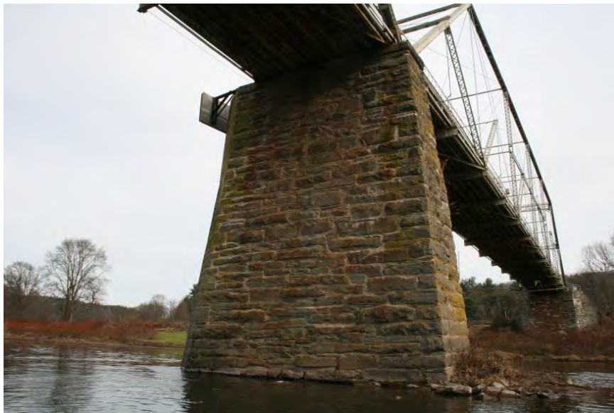
Photo 28- Skinnners Falls Bridge: Sediment Island with Vegetation Downstream of Pier
