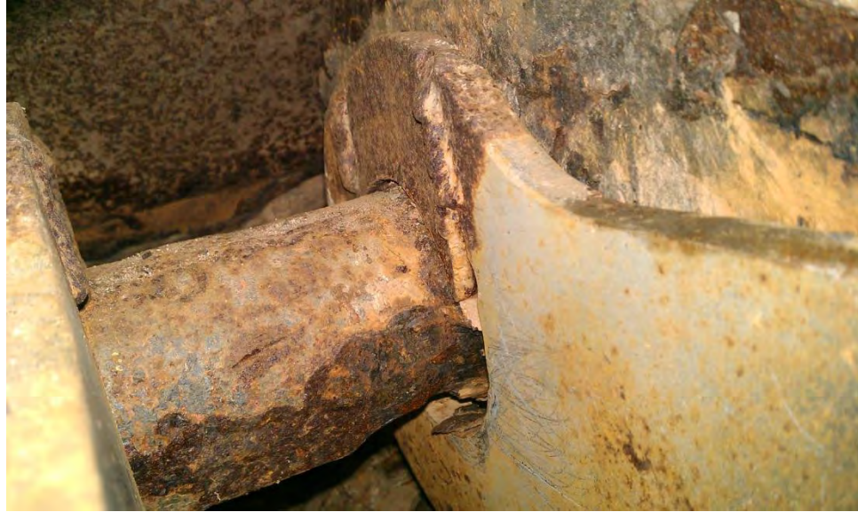
Photo 15 - Skinners Falls Bridge: 1/4" Section Loss to one side of pin at Span 1, Left Truss, Panel Point L0 (Looking Back)
