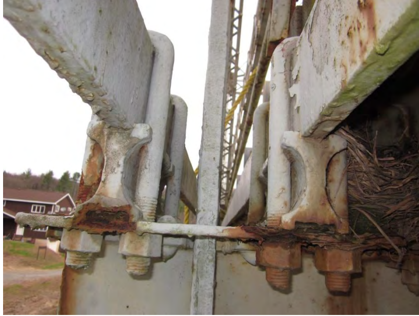
Photo 21 - Skinnners Falls Bridge: Floor Beam Support deterioration
