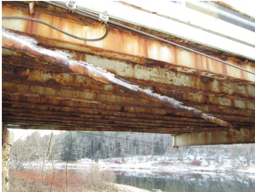
Photo 22 - Skinnners Falls Bridge: Span 2, Floor Beam Bay 12, 100% section loss to bottom lateral bracing
