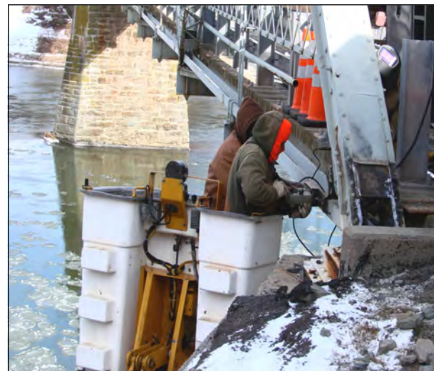
Workmen at the bridge in January 2010. Despite frigid conditions they soon finished the job. Note ice on the Delaware River.
