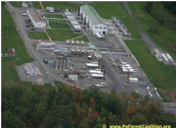
Compressor Station in the Susquehannock State Forest
