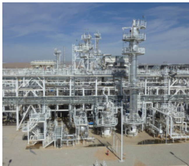
Natural gas processing plant
