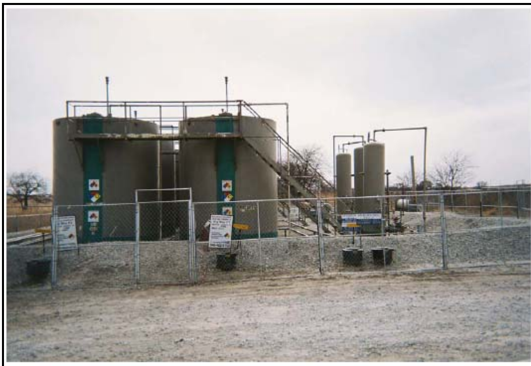
Figure 5. Example Storage Tank Battery (left), Separators (right), and Piping. (14)
